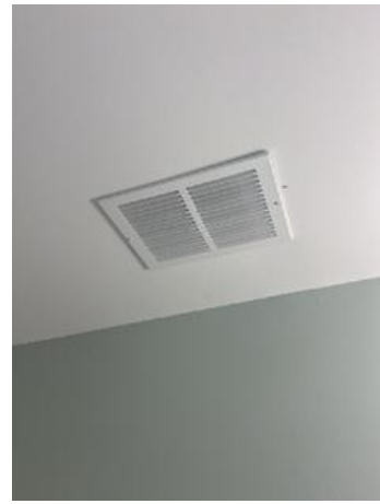
Exhaust Fan 📅 2024-03-07 15:00:22 🔍 30.71852751544743, -88.27530909337874 🖼️ Image
